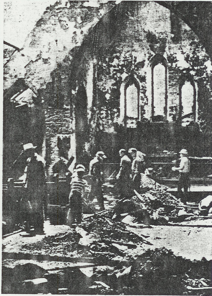
RUBBISH CLEARED AWAY —Saturday was a busy day at the Trinity Episcopal Church as about 22 men helped clear away part of the rubbish resulting from the church's $114,000 fire. Rev. Robert Swift said final plans are being prepared by the architect, with construction due to start sometime in September. (Journal-World Photo.)
